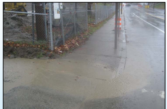
Sediment-filled runoff from a construction site
